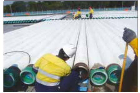
PIPES ADMINISTERED WITH VpCI
