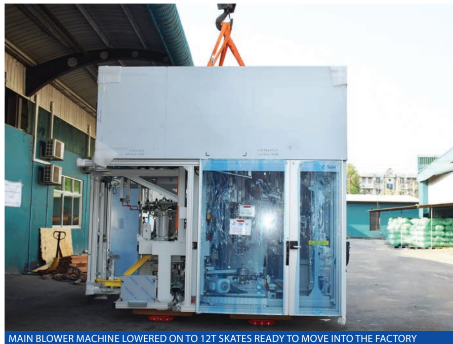
MAIN BLOWER MACHINE LOWERED ON TO 12T SKATES READY TO MOVE INTO THE FACTORY
