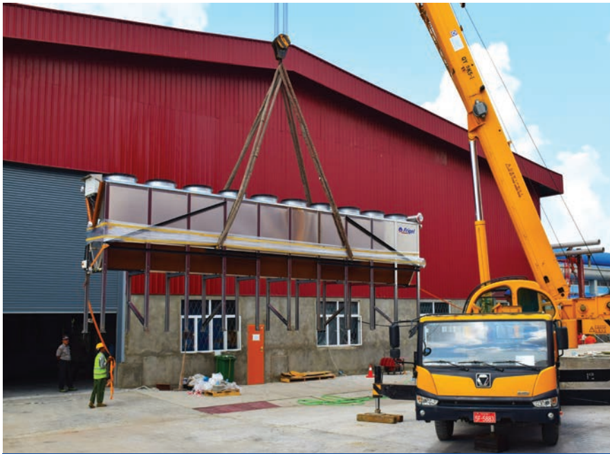
HEAT EXCHANGER WITH LEGS ATTACHED LIFTED INTO POSITION WITH A 30T MOBILE CRANE
