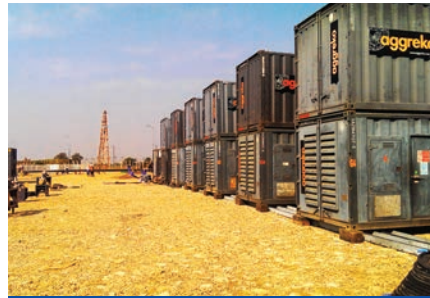
GENERATOR SETS DOUBLE STACKED ONSITE
