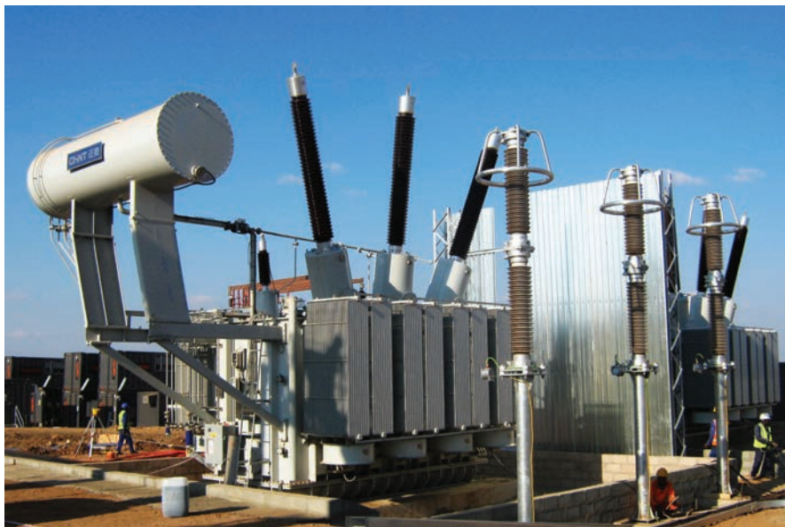
SITE SUBSTATION COMPLETED AND READY FOR HOOK UP
